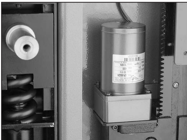
Figure 95. Guide post elevation motor wiring.
